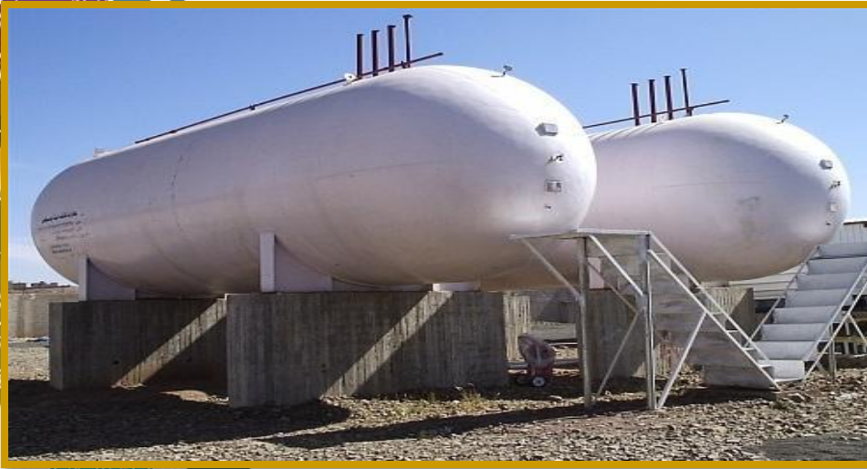
AMMONIA STORAGE TANKS
