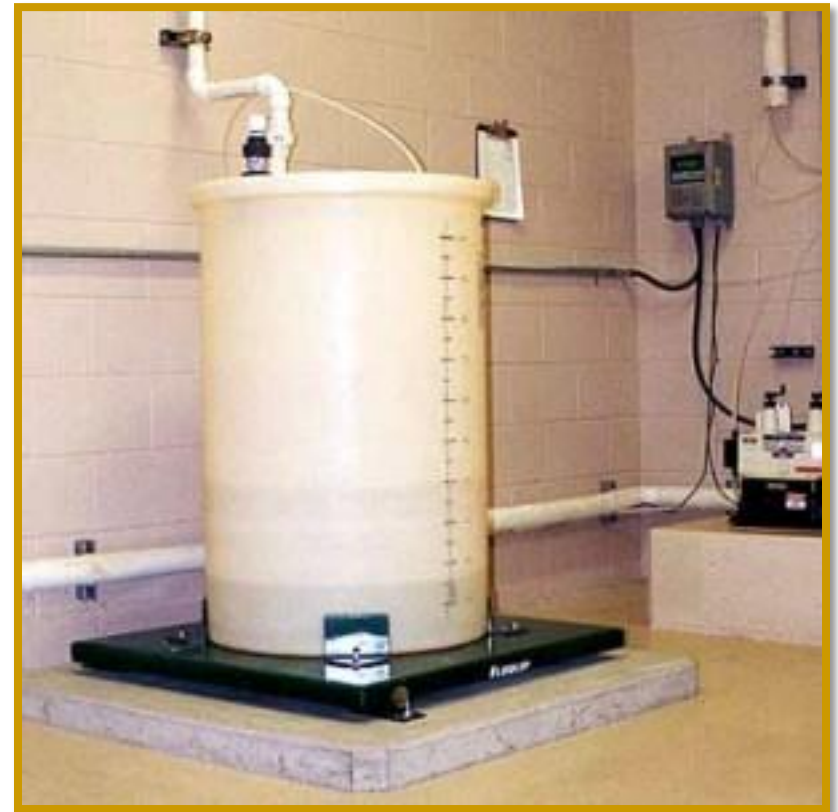
CHLORINE FEEDING TANK
